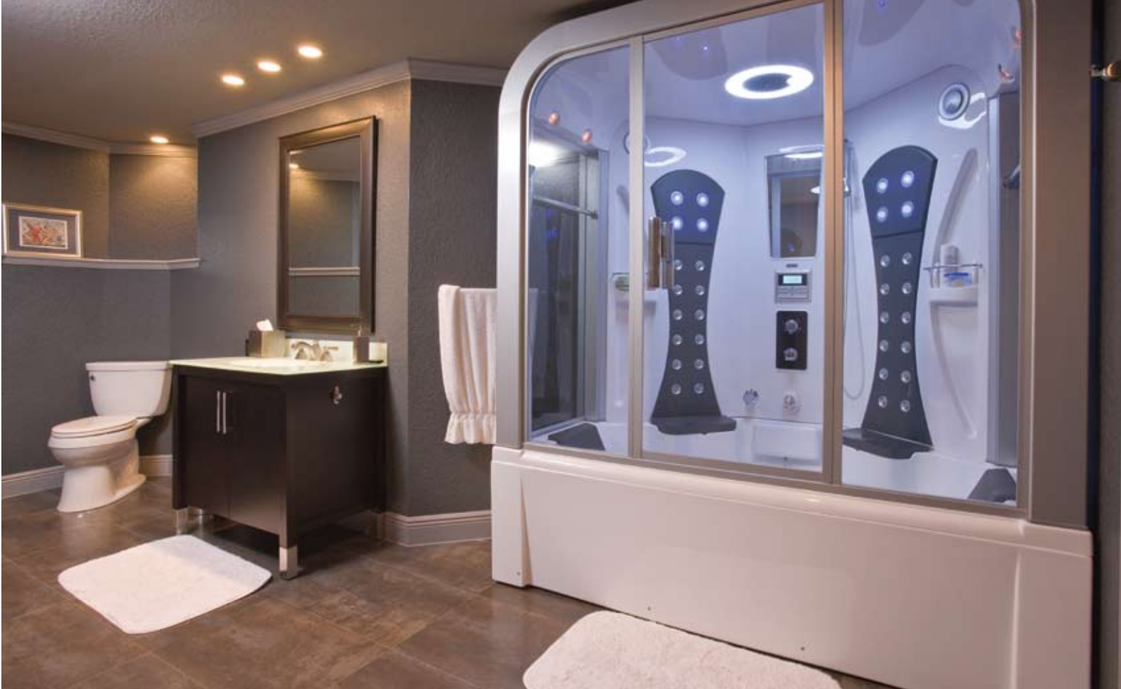
This special-order shower needed to be assembled in place because of the size of the room. The unique unit includes horizontal jets, a built-in radio system with speakers, a spa and a steam bath.
